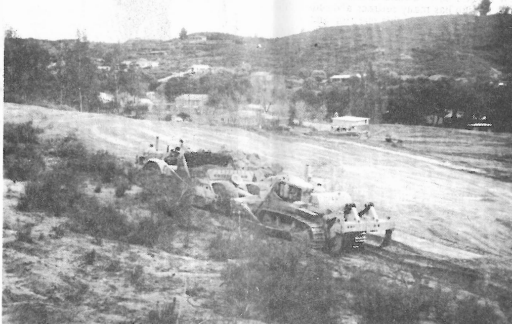
Heavy dozer on site for new trailer park pushes giant earth scoop in leveling ground and making fills which Contractor Paul Pullaro uses here. Photo is southeast toward Hwy 80.
